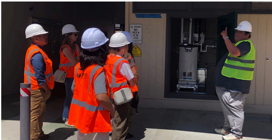
Pictured above is Bond and Program Manager, Eric Van Pelt, showing the new furnaces recently installed at North School during the Citizens Bond Oversight Committee (CBOC) site visit.
